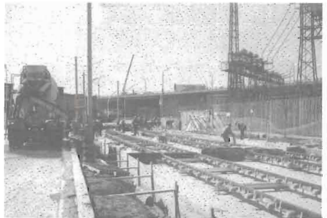
On April 17, 1996, workmen were installing tracks for the TTC's new Eastern Entrance Loop at the Canadian National Exhibition grounds. This view looks northwest west of Strachan Avenue. Photo by John Thompson.
